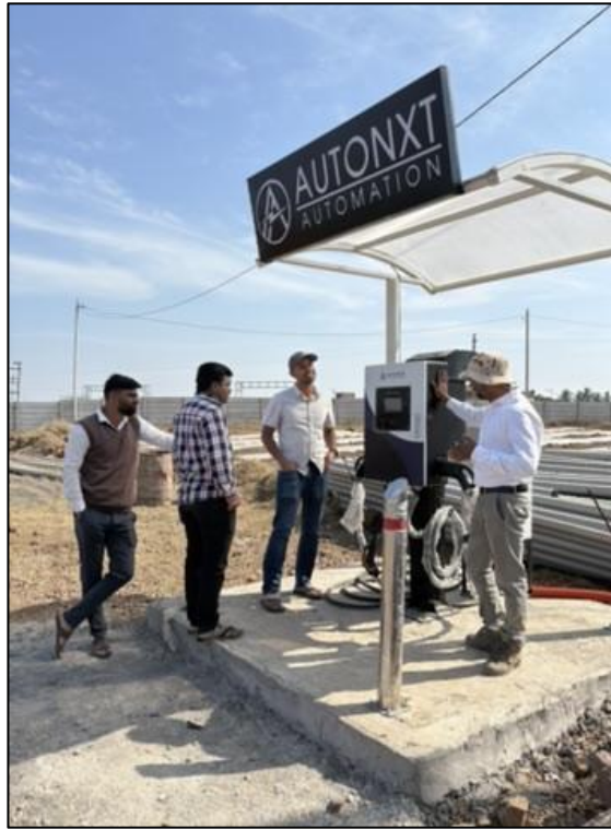
Community on-farm charger
